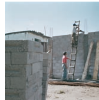
Page 23: Building a new house for a villager who is still in the United States, Tonalapa, 2008.
